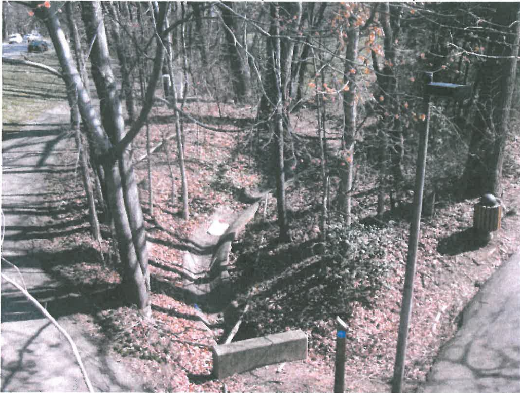
23. Looking east (downstream) at a concrete-lined ditch on the Lake Anne study area. This feature does not provide suitable habitat for wood turtles. (Attachment 1, Sheet 3)
